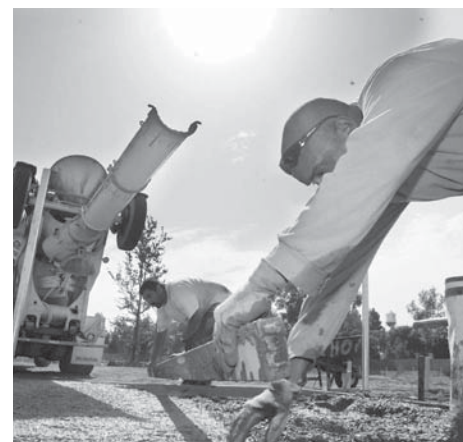
Raul Romero, left, and Caesar Yslas, both of Swinerton Builders Concrete Services, volunteer by paving the dugout with concrete.
