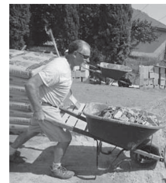
Randy Worrel, a volunteer from Home Depot, moves a barrel of debris from the construction area. "What a blessing it is to do something for the kids," he said.
