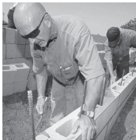
Mike Thelen and Richard Knowlton clean up excess concrete from bricks in a wall at the baseball field.
